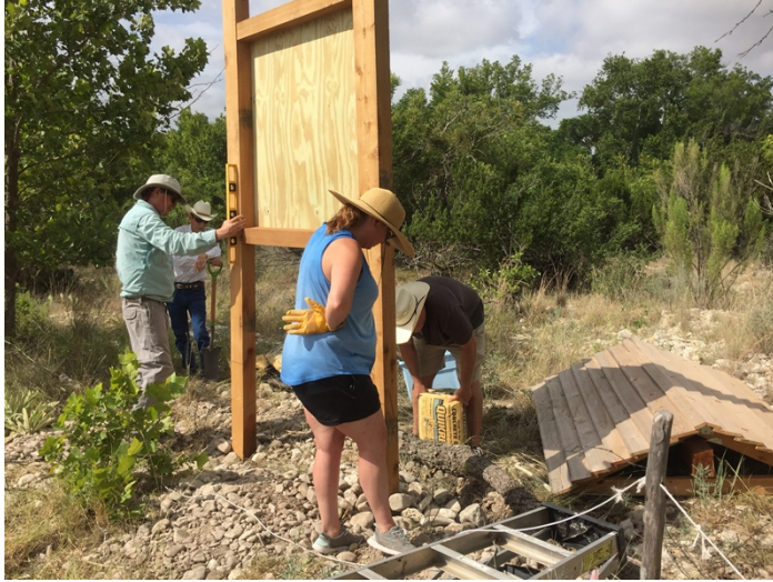
Volunteers install and level sign kiosk under the watchful supervision of Board Member Art Mudge
