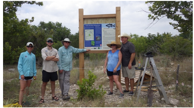
Mission Accomplished – well almost. Kiosk roof to be added once concrete sets.
