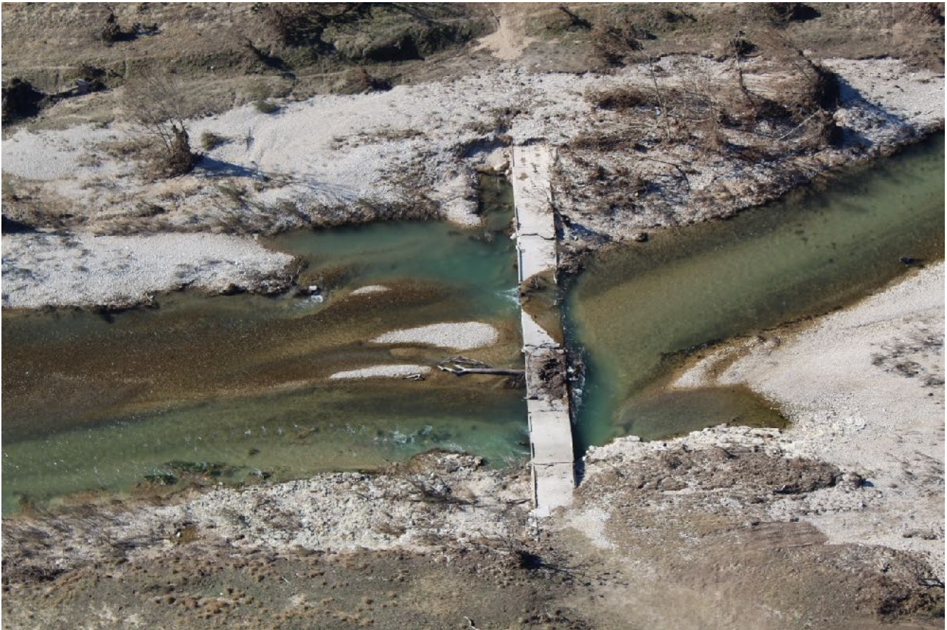
Figure 26. Collapsed Bridge at Kimble County Road 310. Boaters must line unlined boats along swift current on river left (bottom)
